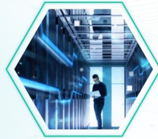
Communications & Computing (C&C) Business Unit
