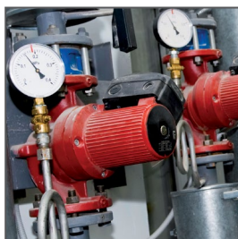
Sensors, valves and control cabinets
